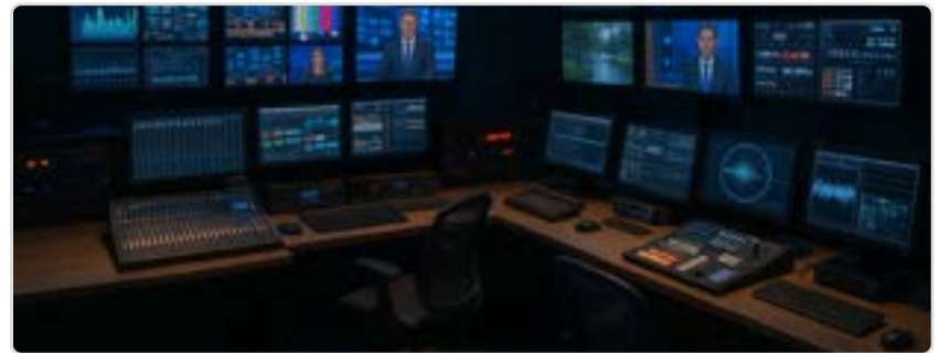
Broadcast Control Center
